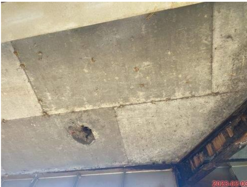
PHOTO 14: MINOR SPALLS IN SOFFIT AT DRAINS (TYPICAL)
