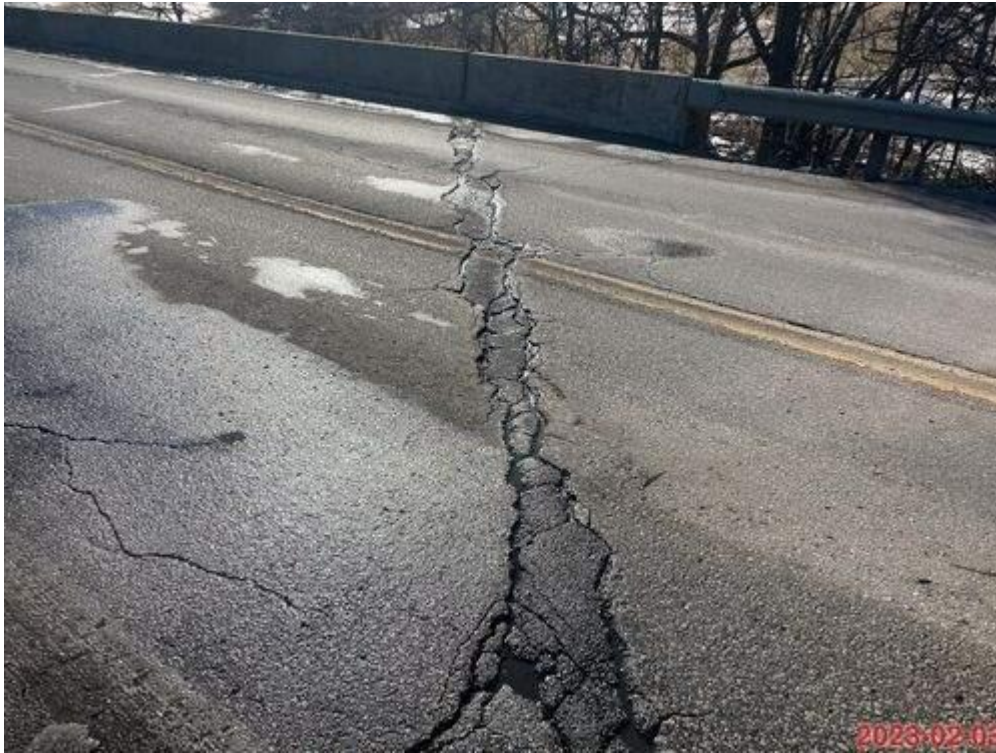
PHOTO 7: DECK AT NORTH ABOUTMENT (TYP AT SOUTH) – CRACKS, SPALLS, AND PATCHES
