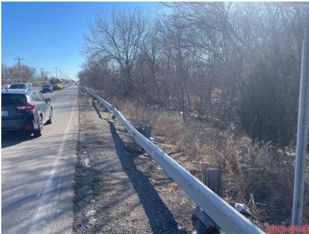
PHOTO 6: RAIL DAMAGE (TYPICAL)
