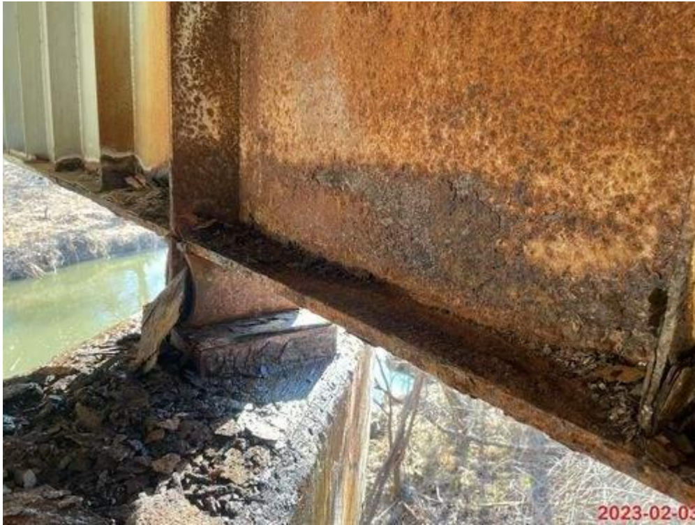
PHOTO 13: BEAM 1 AT PIER 2 – 15% SECTION LOSS
