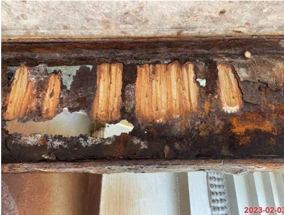
PHOTO 15: DIAPHRAGMS AT PIER 1 HAVE MODERATE TO HEAVY SECTION LOSS (TYPICAL)
