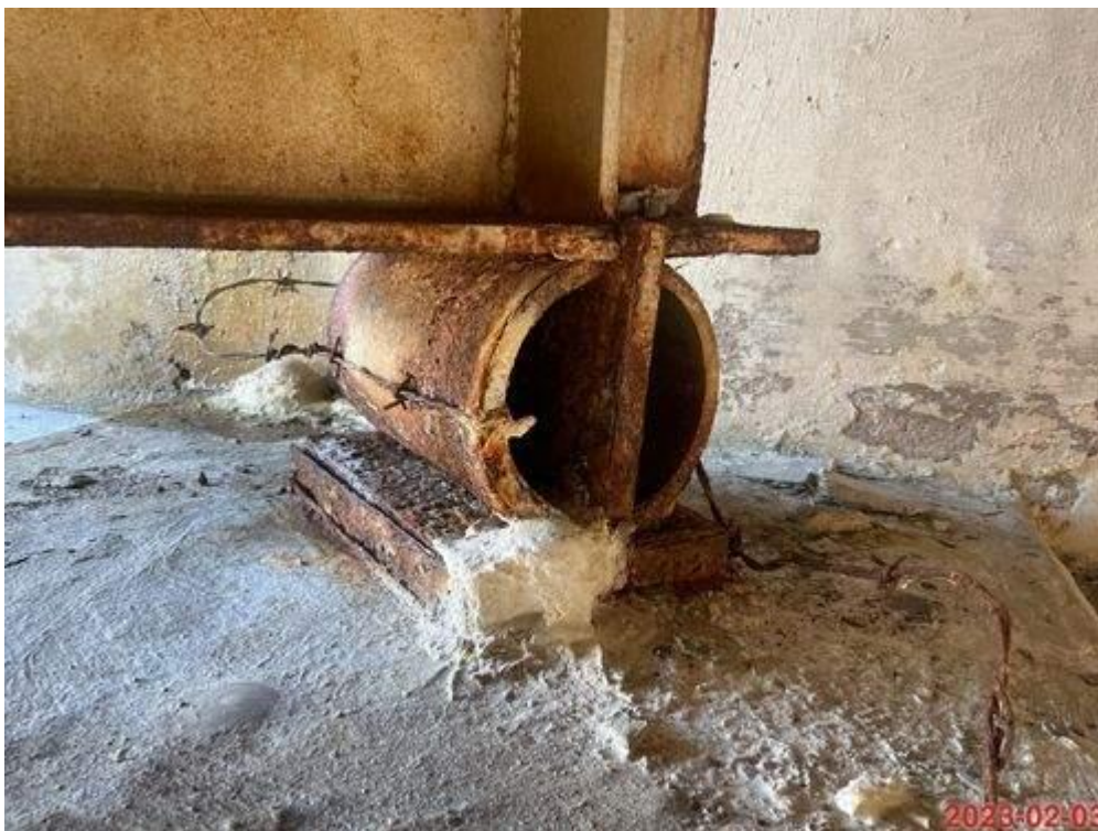
PHOTO 18: BEARINGS AT ABUTMENTS HAVE HEAVY CORROSION (TYPICAL)
