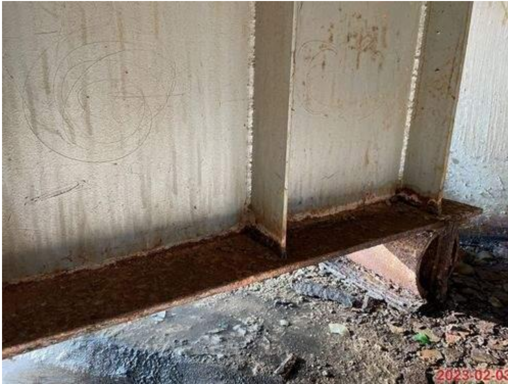
PHOTO 9: BEAM 1 - MINOR SECTION LOSS OF BOTTOM FLANGE AT NORTH ABUTMENT
