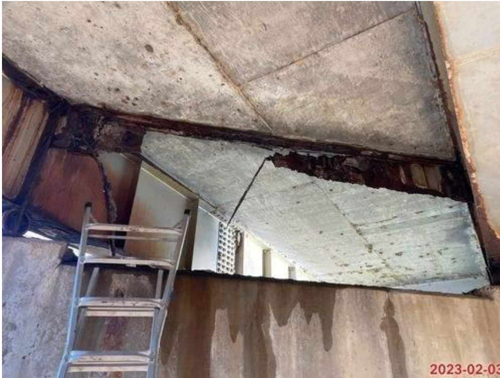
PHOTO 11: DIAPHRAGMS AT PIER 2 HAVE 100% SECTION LOSS (TYPICAL)
