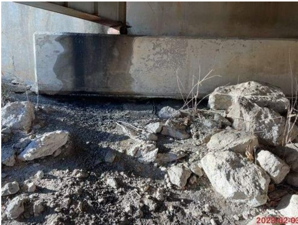
PHOTO 10: NORTH ABUTMENT - EROSION WITH EXPOSED PILES
