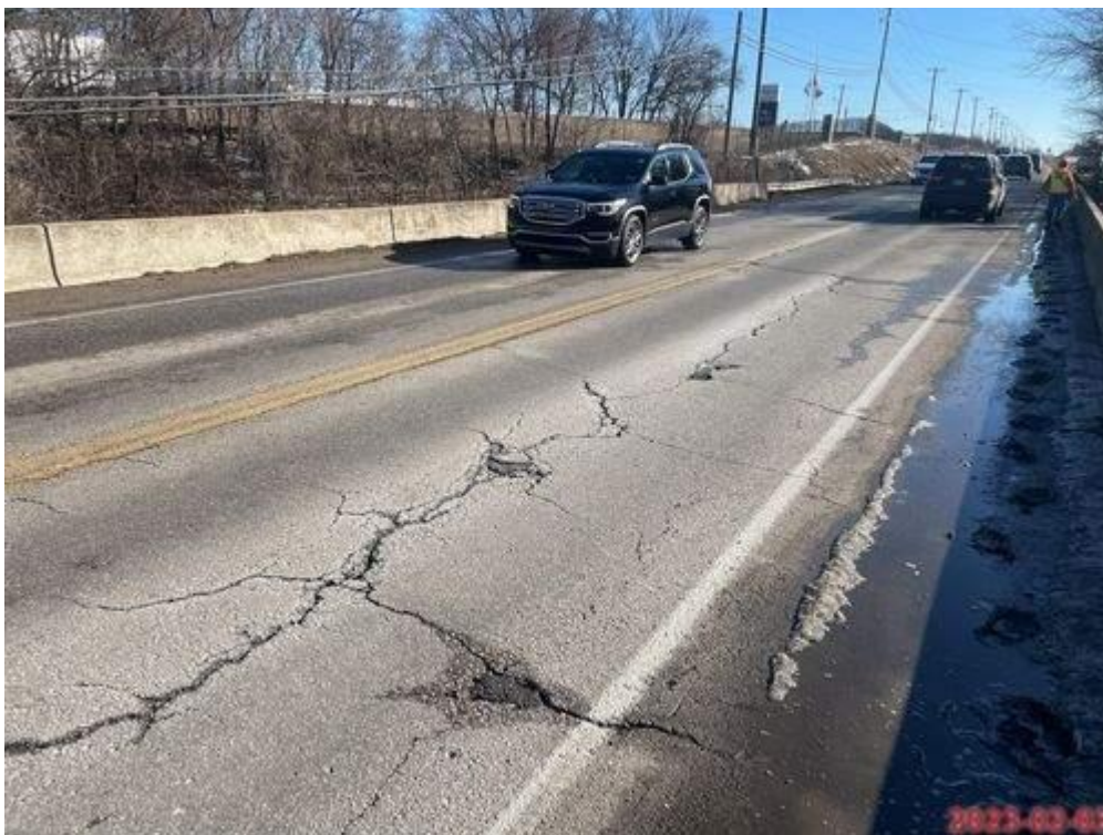
PHOTO 8: DECK WITH POTHOLES AND CRACKING IN OVERLAY
