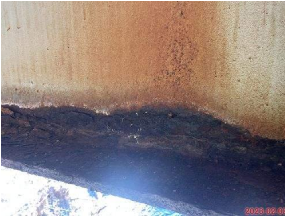
PHOTO 17: BEAM 1 AT PIER 1 – MODERATE SECTION LOSS
