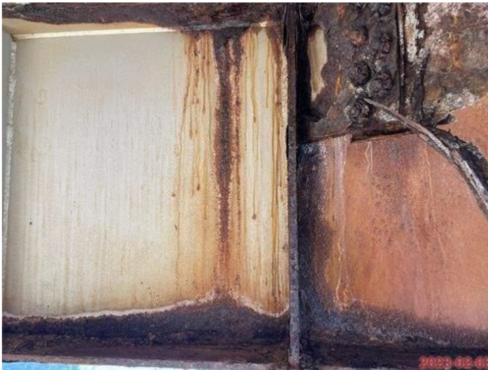
PHOTO 12: BEAM 4 AT PIER 2 – 15% SECTION LOSS
