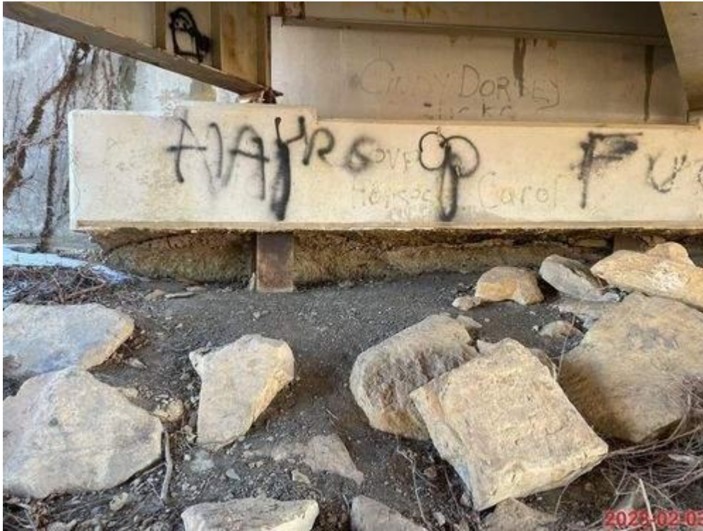
PHOTO 21: SOUTH ABUTMENT UNDERMINED 24"
