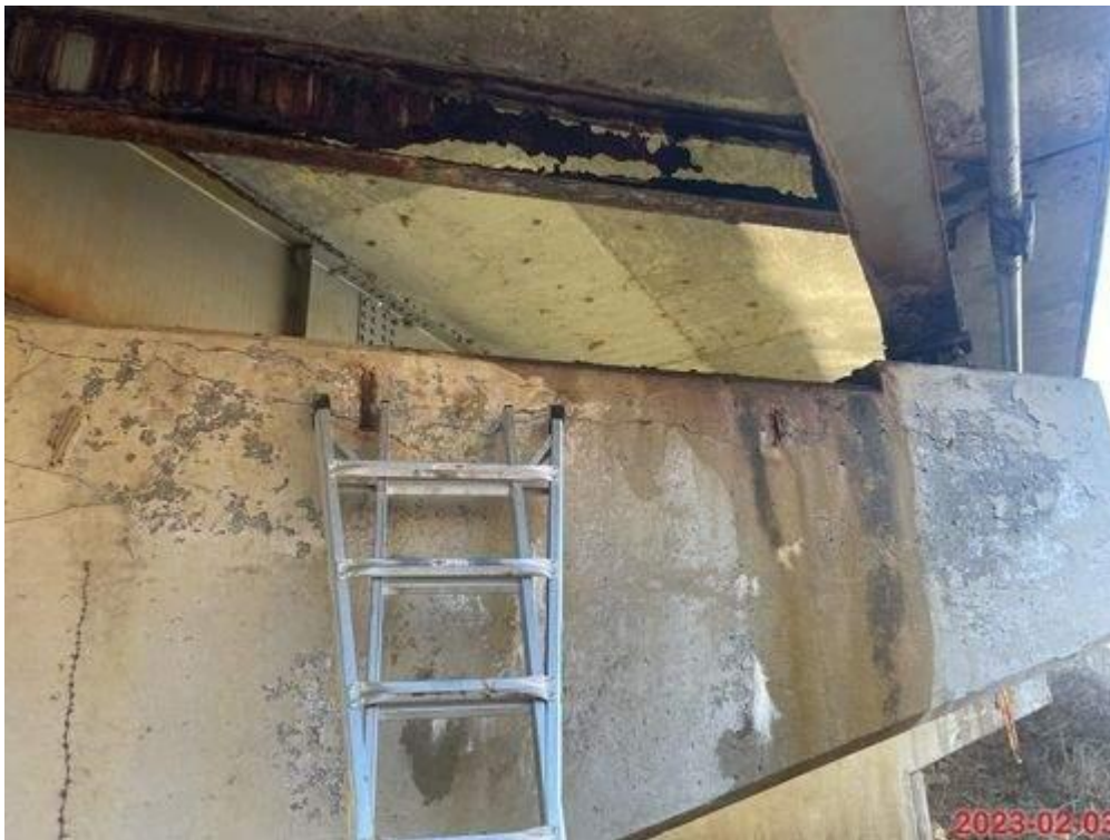
PHOTO 20: PIER 1 MINOR SPALL AND DELAMINATION SOUTH FACE (TYP)
