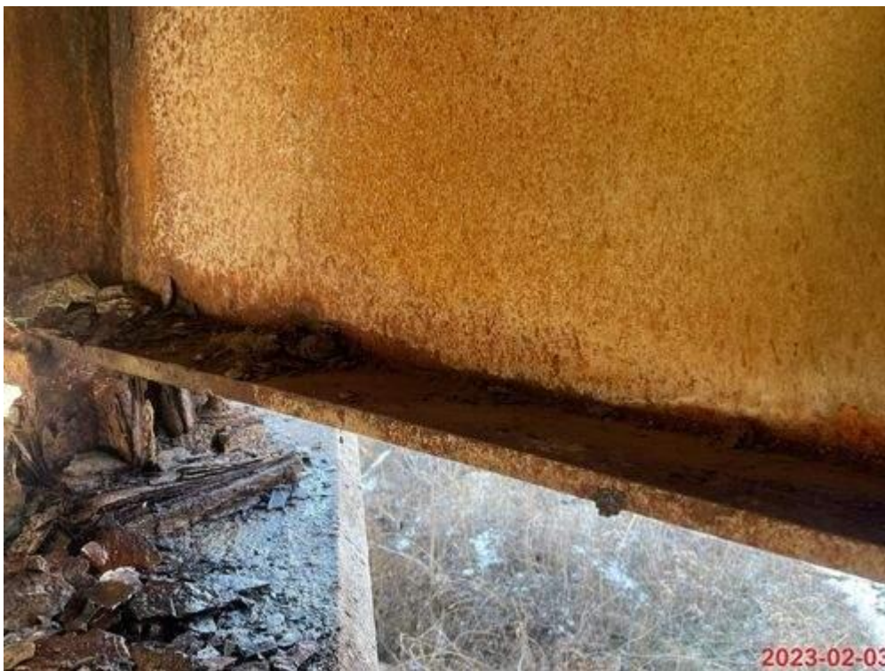
PHOTO 16: BEAM 4 AT PIER 1 – MINOR SECTION LOSS
