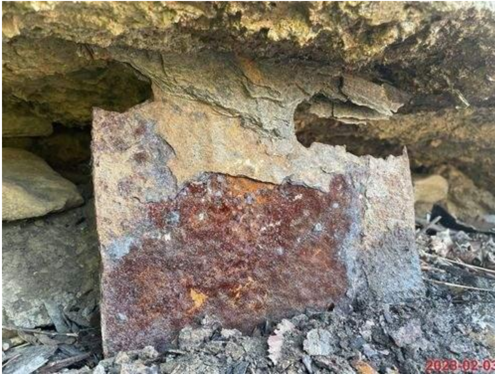
PHOTO 19: PILE 1 SOUTH ABUTMENT FLANGE RUSTED THROUGH WITH 35% SECTION LOSS
