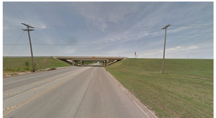
No sidewalks under the Creek Turnpike
