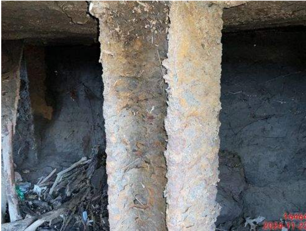
PHOTO 7: WEST ABUTMENT SCOUR - TYPICAL EXPOSED STEEL PILE
