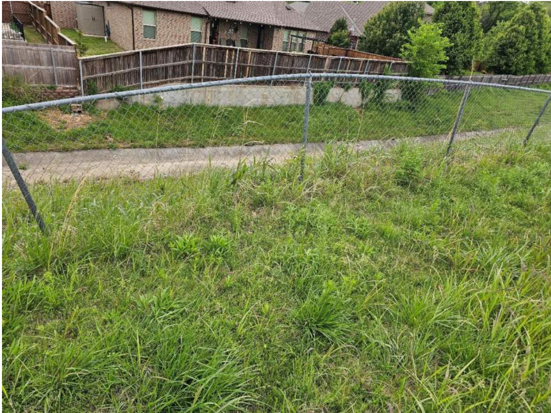
Section of fence not fallen for reference.
