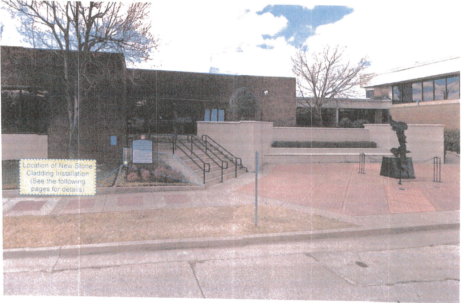
151703B - City Hall Renovations - Entry Plaza Planter Wall COR 01 Drawing Mark Up - 10/10/2016
