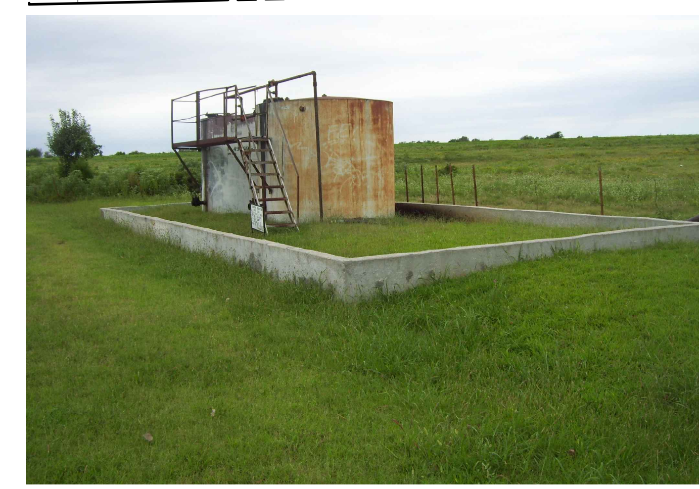
EXISTING OIL TANKS AND CONCRETE RETAINING WALL ALONG WASHINGTON STREET APPROXIMATELY 2,560' EAST OF S. 9th ST.
