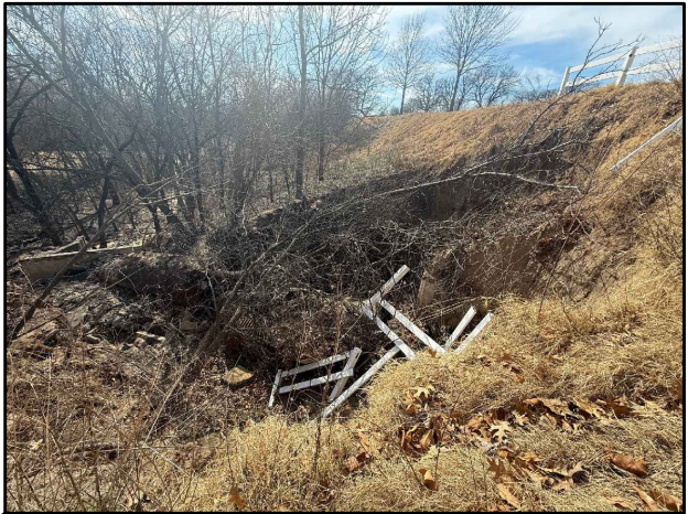
PICTURE 1: EXTENTS OF EROSION ALONG SLOPE
