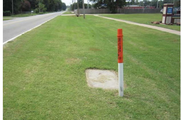
Fiber Optics Utility at Kingdom Hall of Jehovah's Witnesses - Looking south
