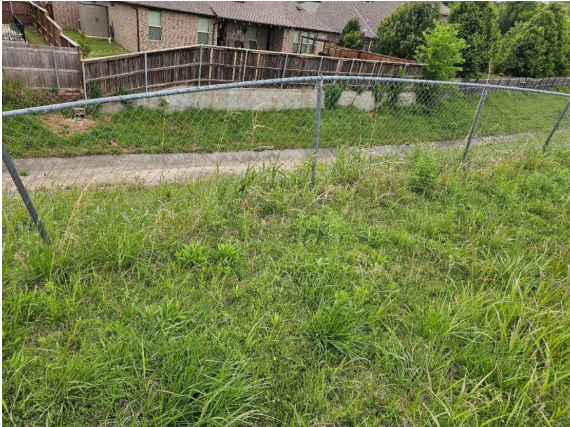
Section of fence not fallen for reference.
