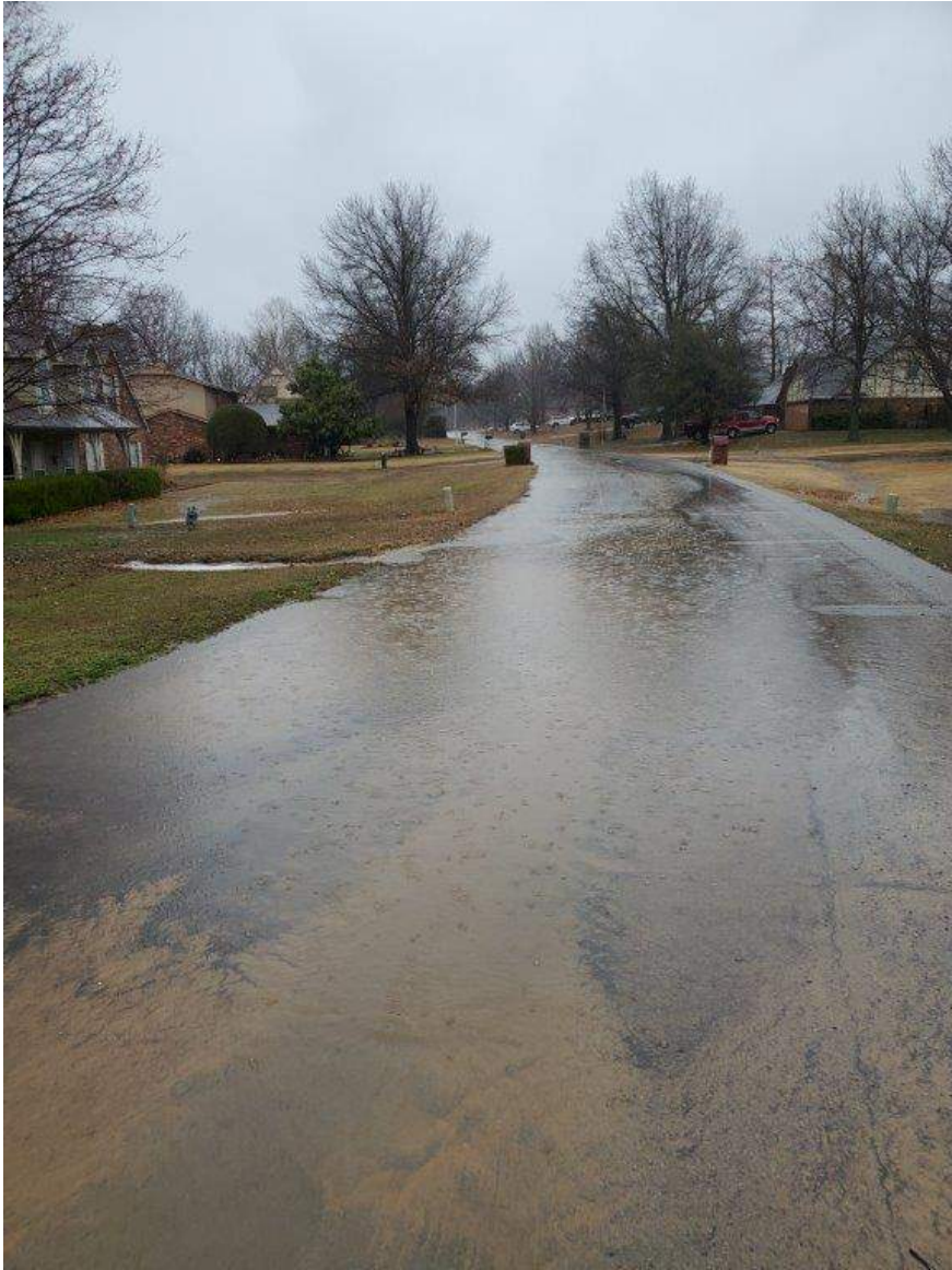
Low spot on the road – S. Harp Blvd.
