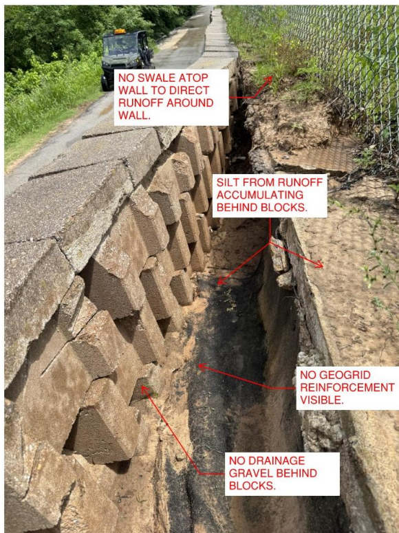
Figure 1: Bulge in wall
