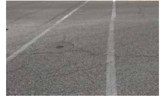
Poorly marked cross walks on New Orleans.
