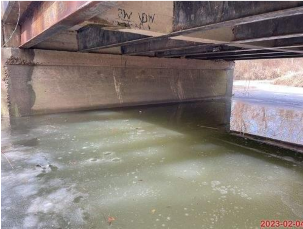
PHOTO 7: WEST ABUTMENT - MINOR CRACKS AND SPALLS
