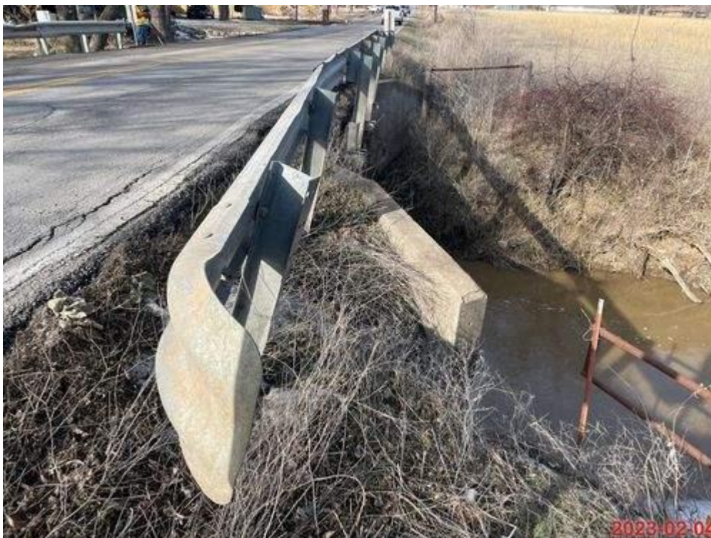
PHOTO 6: SE CORNER EROSION (TYPICAL)
