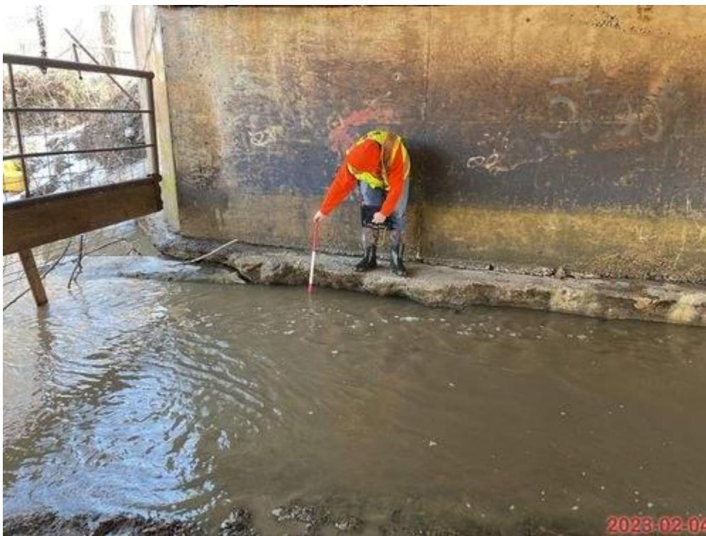
PHOTO 10: SOUTH ABUTMENT AND SE WING - UP TO 30" OF EXPOSED FOOTINGS
