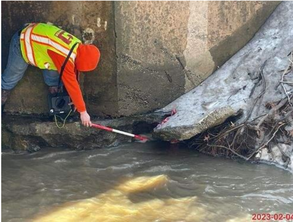
PHOTO 9: SW WING - 12" UNDERMINING
