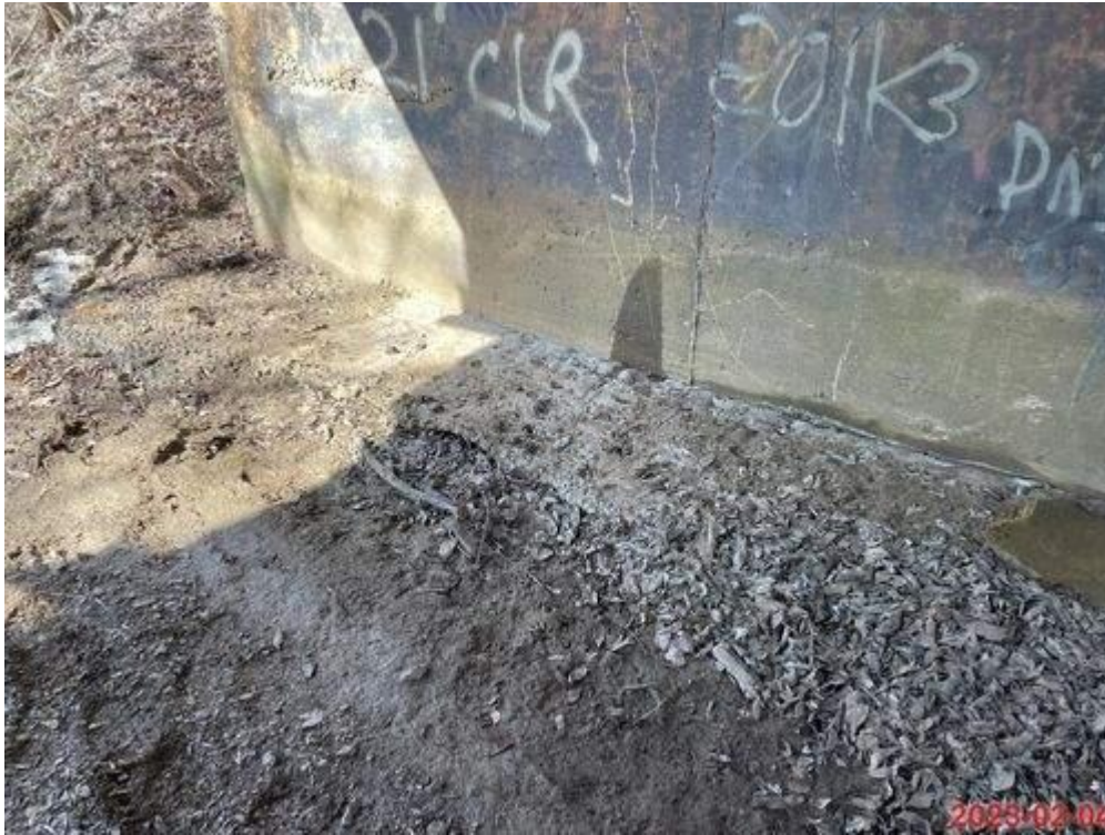
PHOTO 13: NORTH ABUTMENT - EXPOSED FOOTING 6"
