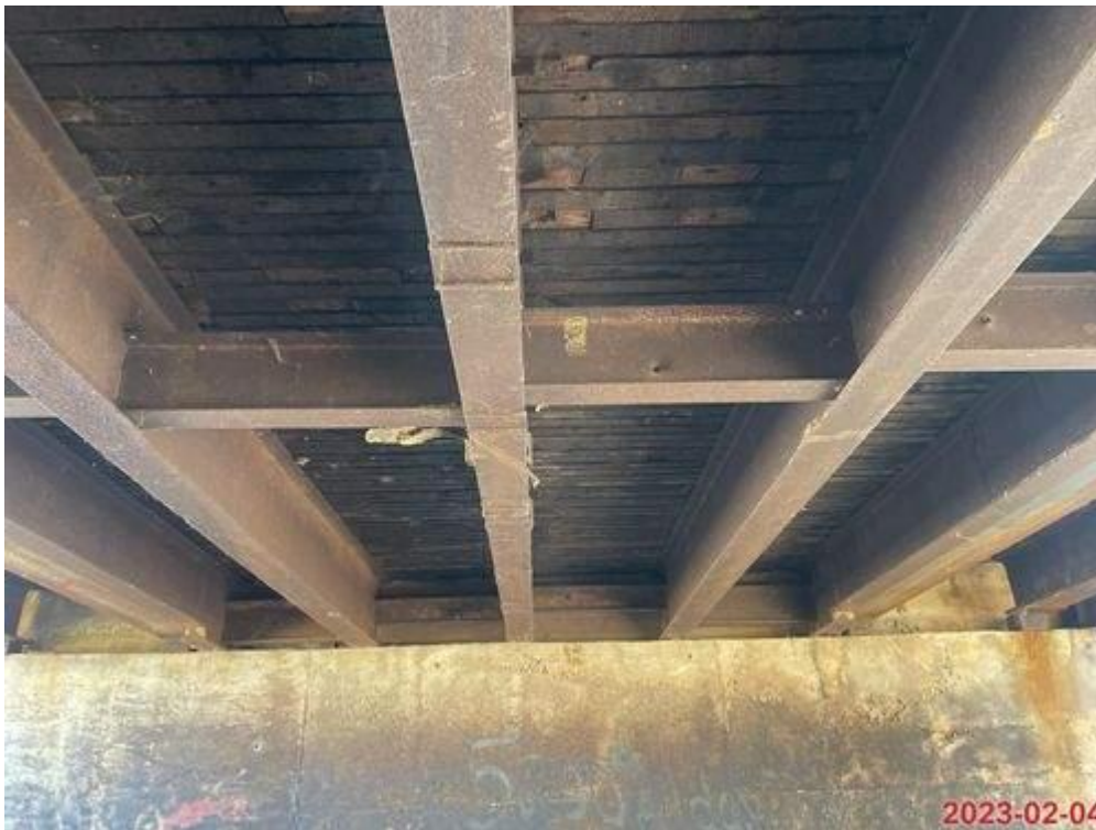
PHOTO 12: BEAMS - MINOR CORROSION
