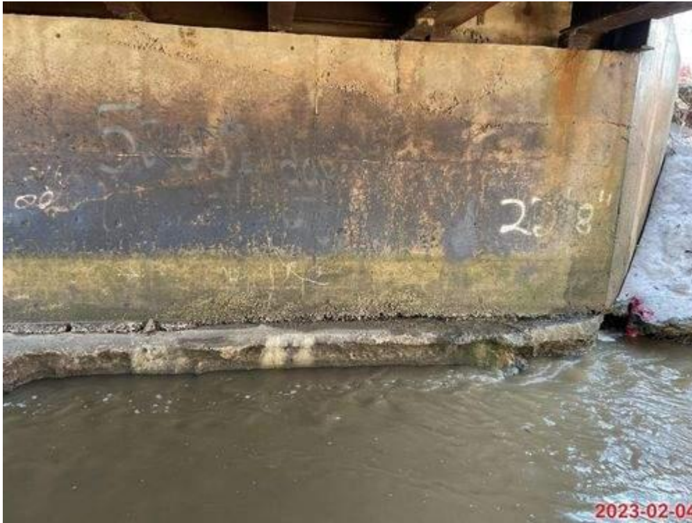
PHOTO 11: SOUTH ABUTMENT - HONEYCOMB (TYPICAL)
