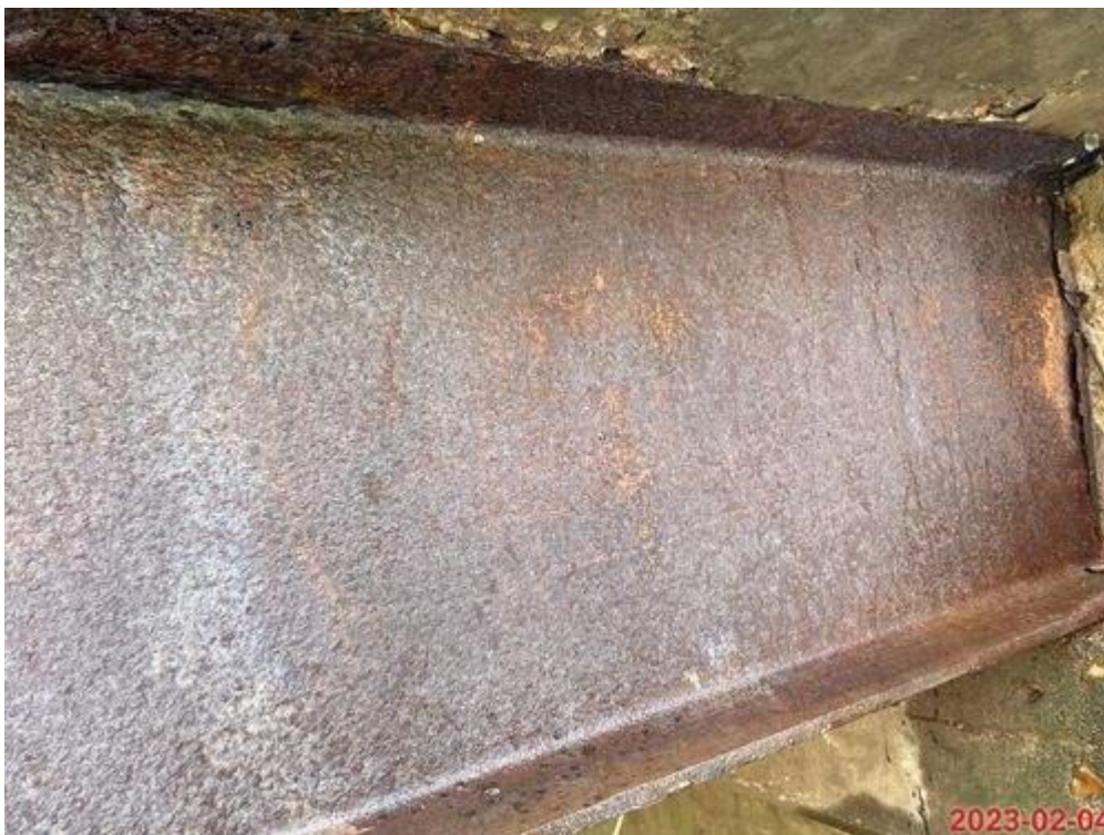
PHOTO 6: GIRDER 7 AT ABUTMENT 2 – MINOR SECTION LOSS
