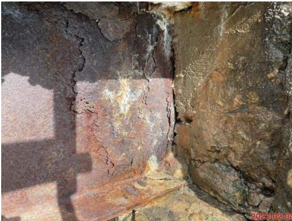
PHOTO 8: GIRDER 7 EAST ABUTMENT – MINOR SECTION LOSS
