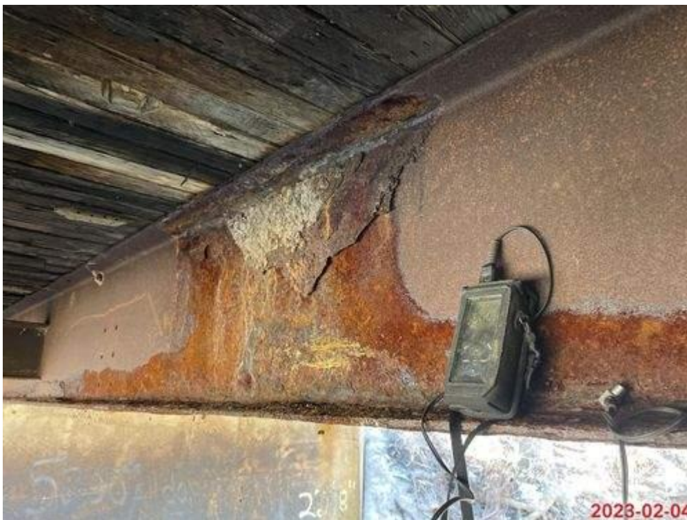
PHOTO 8: BEAM 7 – 4' SECTION WITH MODERATE SECTION LOSS UP TO 50% IN BOTTOM FLANGE AND 33% IN WEB
