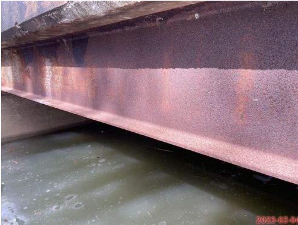
PHOTO 9: TYPICAL GIRDER CORROSION
