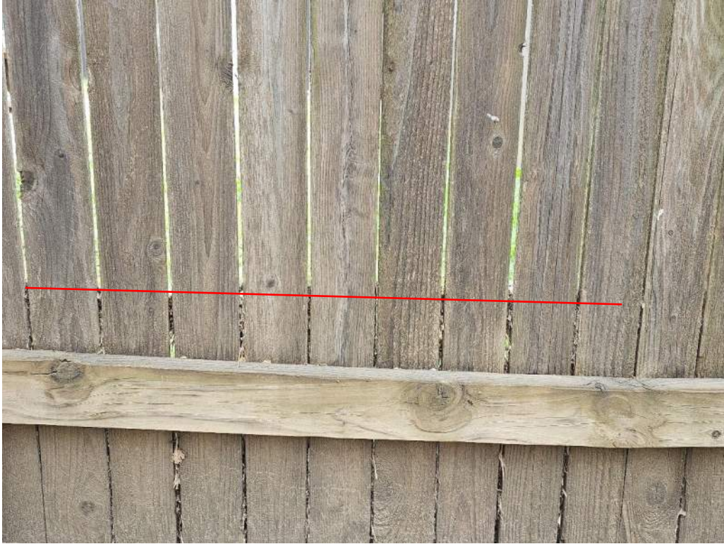
Debris line along fence
